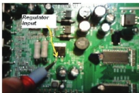
Checking Input Voltage to Regulator
